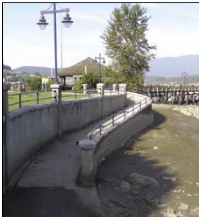
Beach Access Ramp – Rocky Point, Port Moody, B.C. photo credit: Petra Frederick
