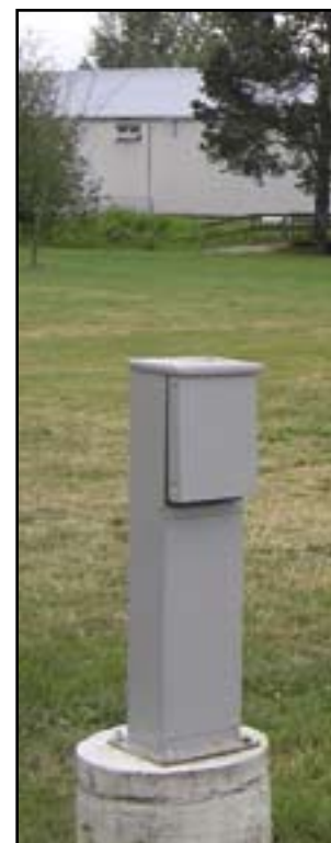
Battery Recharge Outlet – Maple Ridge Fairgrounds, Maple Ridge, B.C. photo credit: Donna Rodman
